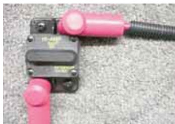
Figure 4-7. Main Circuit Breaker
