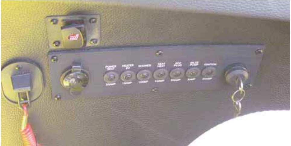
Figure 2-13. Circuit Breaker Panels
